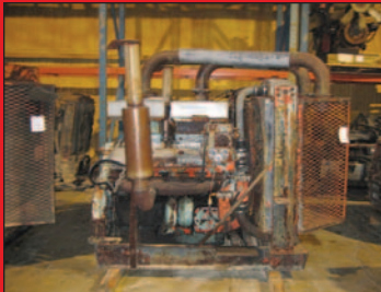
Detroit 12 V 71 Power Unit
