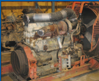
Cummings KTA 500 HP Power Unit
